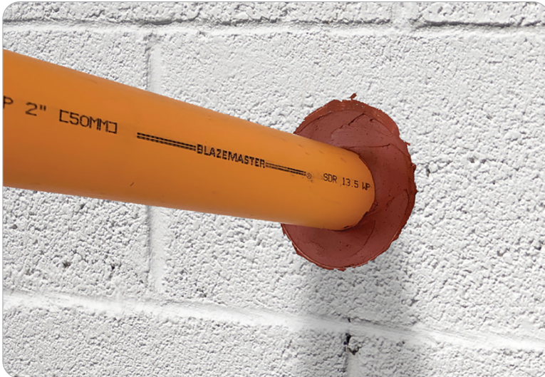
2-Hour Fire-Rated Through Penetration Firestop for Single Plastic Pipe through Concrete Walls using BlazeMaster Caulk & Walk.
